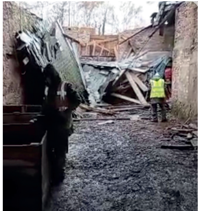
Figure 12, Image of worker amongst dangerous farm infrastructure.
