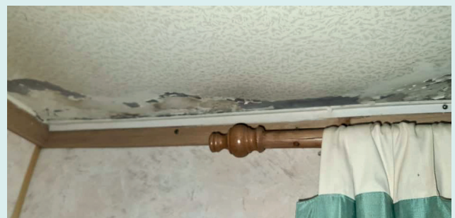
Figure 21, Damp and mould in caravan.
